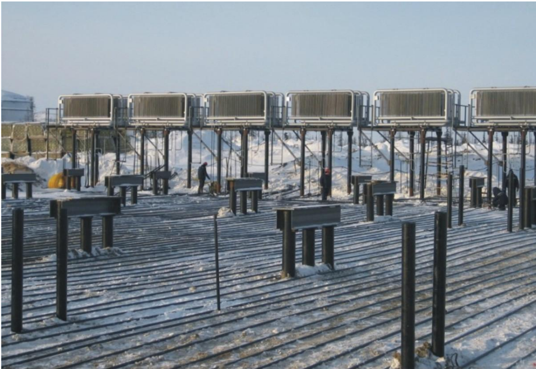
Figure 9. Assembling tubular thermal stabilization system for permafrost soils in foundation of industrial facility
