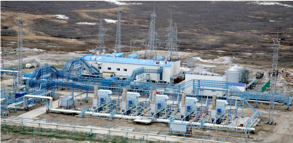
Figure 5. Captive power plant at production site No. 1
